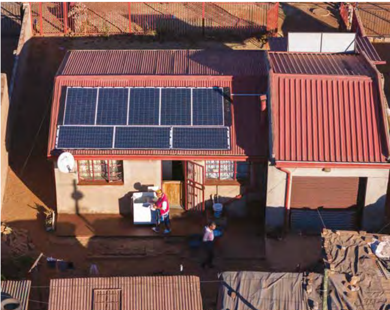
Installed Wetility solar
