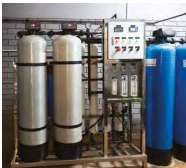
Water purification system
