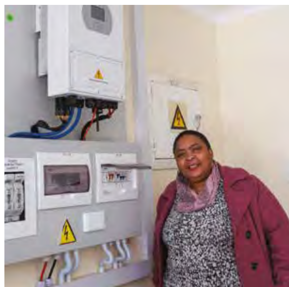
Clean energy system
