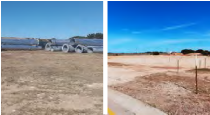
Bulk HV Electrical Installation in Zone 2, Coega SEZ.
