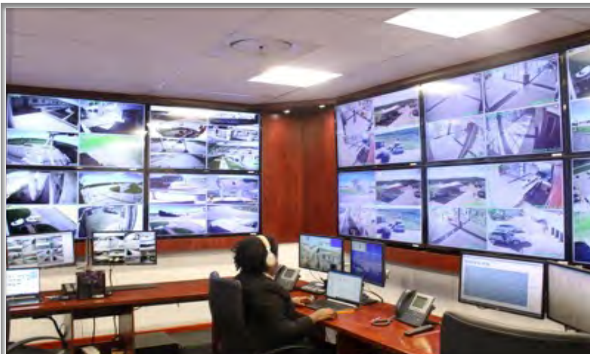
Coega SEZ's Command and Control Centre
