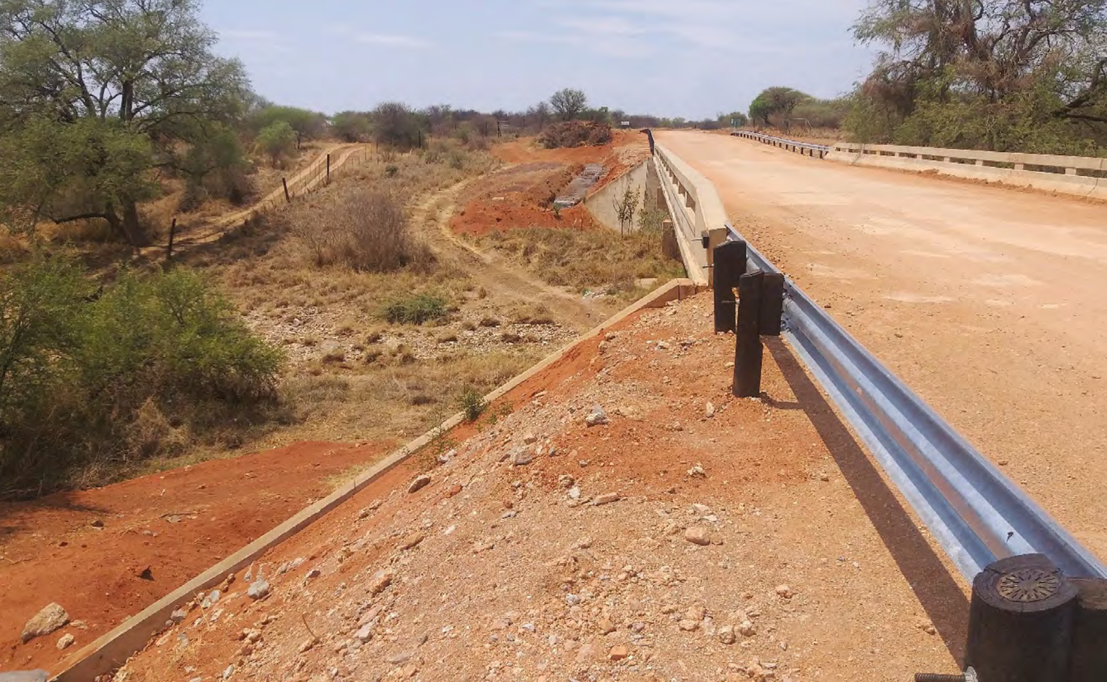
Flood damage repairs conducted in the 2022/23 financial year on a bridge along road D506 that traverses through game farms located between Waterpoort and Musina.
