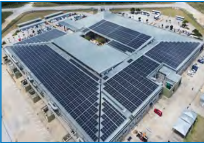
Roof top solar panels have been installed at the Coega SEZ buildings, starting with Business Process Outsourcing (BPO) Park, where Discovery Health Call Centre is located.
