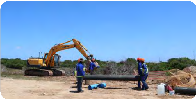
Water & Sewer Infrastructure in Zones 3 & 4
